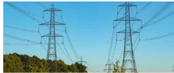
Transmission Lines Across the United States
